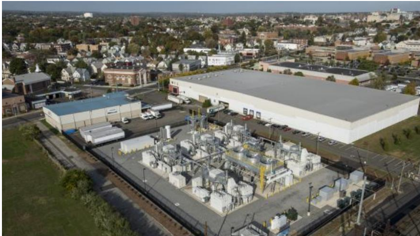
15MW Dominion Bridgeport Fuel Cell Park
